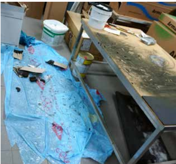
When installing PUR and cellular glass, considerable amounts of dust occur and the working area must always be covered with a tarpaulin.
