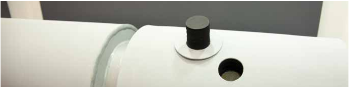
Figure 8. Example of inspection 'port hole' created with FEF insulation materials.
