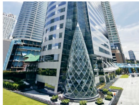
ArmaFlex® was installed on the chilled water system of the Sathorn Square building in Thailand's capital city of Bangkok, to prevent condensation and minimise energy losses.
